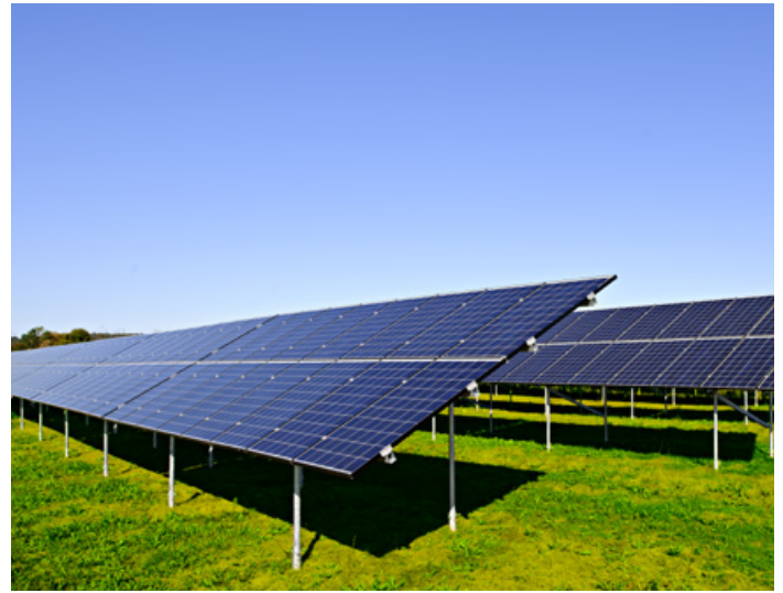
Fig. 3: A clean and functioning solar installation
