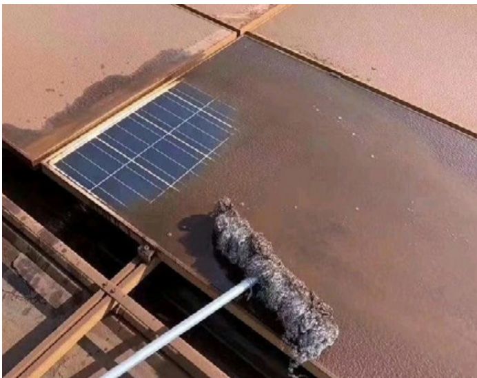
Fig. 2: Dust fall on solar panels.
